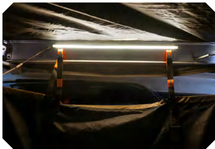
LED light stripembedded in the shower room
